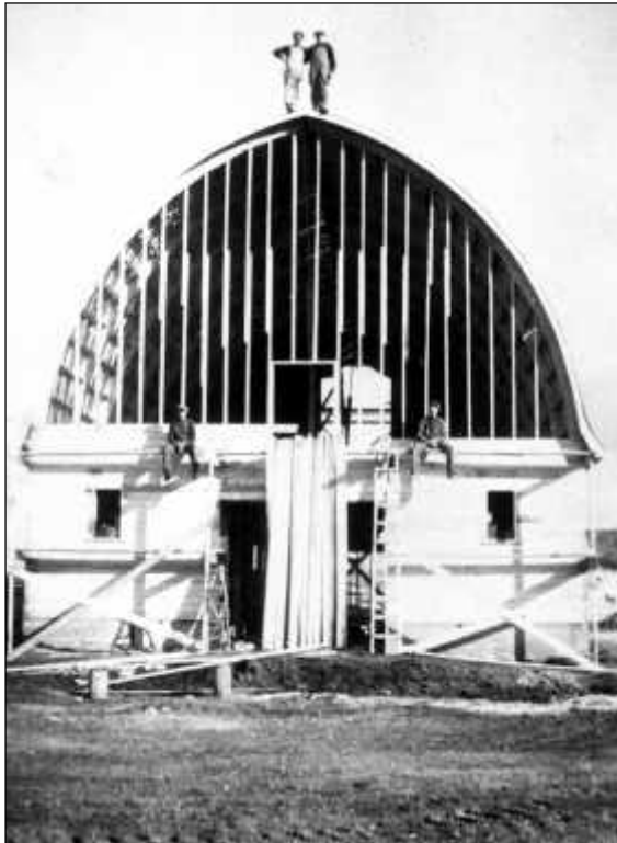
Above: Mr. John Zasiitko and his wife, Pearl, are having a barn built by Mike Troschuk with the help of their sons, Fred and Bill. Bill Zasiitko and carpenter Mike Troschuk standing on top of the barn, Fred and Peter Zasiitko are on the lower level. The barn was completed in 1945. The loft of this barn was the scene of a number of rollicking barn dances during the late 1940s. The John Zasiitko farm was situated five miles west of Poplarfield. FL-136.
