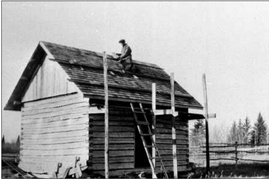
Above: Bill Pawluk putting the finishing touches on repairs to a log building on the family homestead, Broad Valley district, 1930s. The noticeable sag in the old logs and the large horizontal cracks in some of them suggest Bill was not undertaking new construction when this photograph was taken. FL-071.
