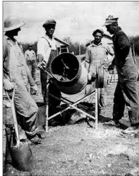
Above: Mixing cement by hand at a construction site at the Philip Horodecki farmstead, High Plains district. L-R: Joe Tycholis, Mr. Horodecki, Anton Pawlowski, Tony Tycholis, Steve Horodecki. FL-128.
