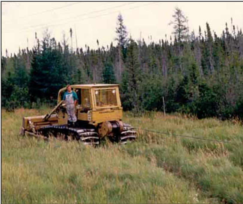
Brian stringing cable with Caterpillar at a job site near Geraldton around 2002.
