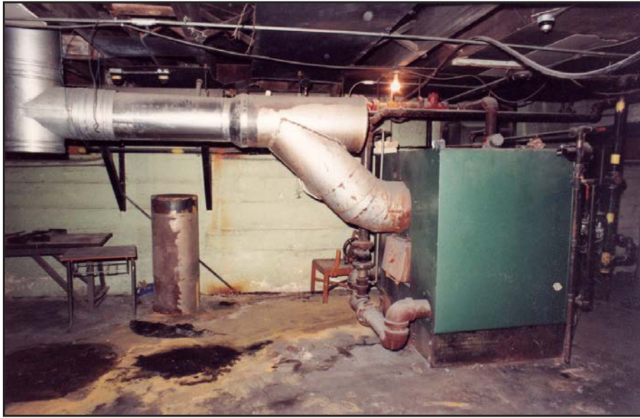
Above. The old fuel oil furnace prior to its removal. ( Heritage Classroom Coll. )
