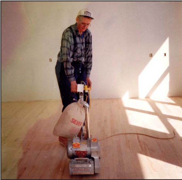
Above. Leo Kristjanson sanding the "new" hardwood flooring, which was salvaged from the old middle school auditorium nearby and installed in the school. ( Heritage Classroom Coll. )
