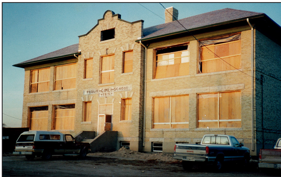
Above. All windows removed, the empty frames boarded over and the building weather tight and secure. Well, almost, some open spaces yet to be covered over. ( Heritage Classroom Coll. )
