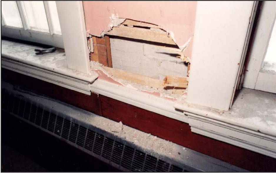
Above. Ripping down the classroom walls. First job, start with a hole. ( Heritage Classroom Coll. )
