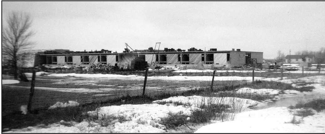
Views of the new Gimli Composite school. Above. Under construction during the early spring of 1961. Below. Soon after completion later that same year. ( Gimli Saga Manuscript, 1973 Pg. 604. )
