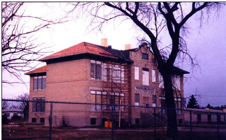
Above. The school building with a scaffold tower set up for the roofers installing a “heritage appropriate” new cedar shingle roof. The old classroom windows were removed at the same time. ( Heritage Classroom Coll. )
