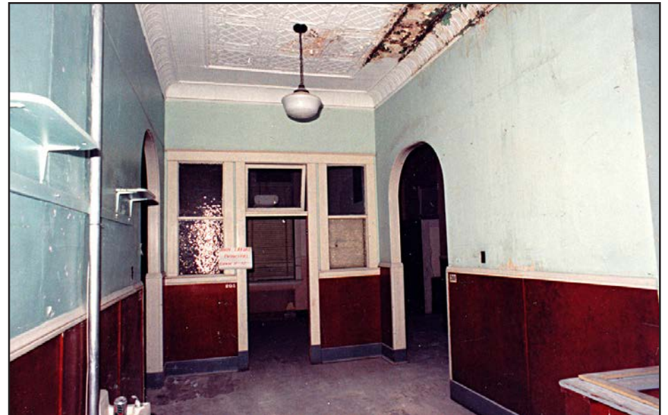
Above. View of the second floor hallway. Note the water damage on the pressed tin ceiling. The handmade sign on the office door frame states: “John Laxdal, Principal Grade 11-12.” (Heritage Classroom Coll.)
