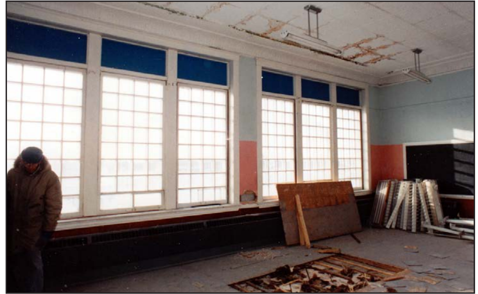
Above. Checking the condition of the floor joists starting with...a larger hole. ( Heritage Classroom Coll. )
