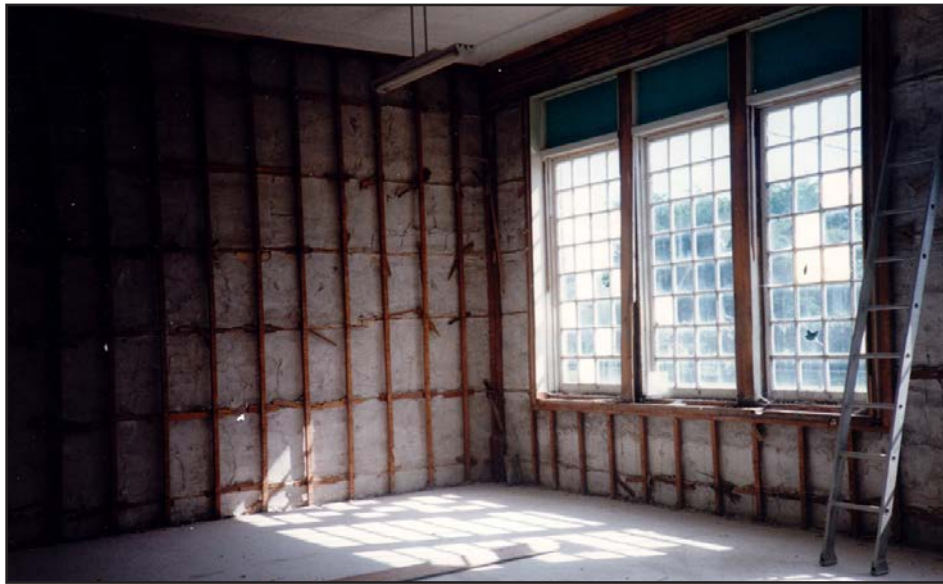
Above. Many, many hours later... bare stud walls with the backside of the brick masonry wall behind them. Note the old windows are still in place. ( Heritage Classroom Coll. )
