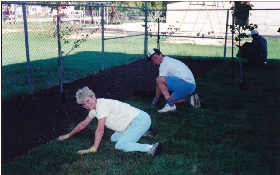
Above. Laying sod on the west side. Chris Brooks in the foreground. ( Heritage Classroom Coll. )
