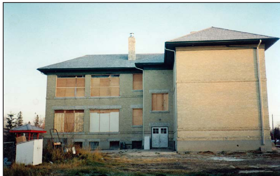
Above. A view of the building from the south, showing about twenty sheets of plywood where windows used to be. ( Heritage Classroom Coll. )
