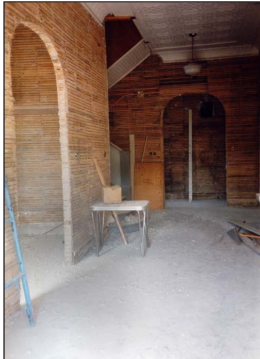
Right. A view of the main level hallway walls after the careful removal of the plaster from the walls without damaging the underlying lath. ( Heritage Classroom Coll. )
