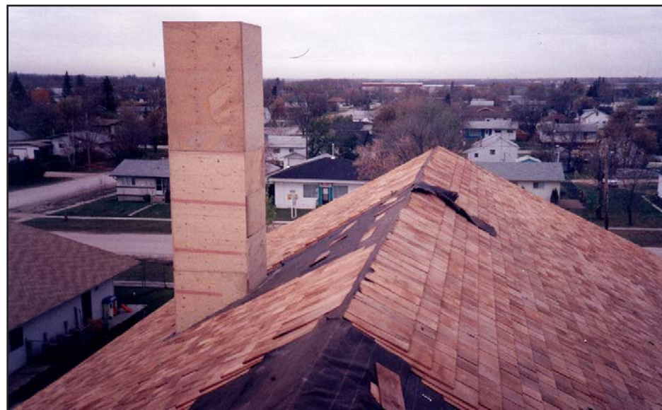
Above. A view of the new wooden shingle roof nearing completion, at least on this wing. Note the plywood protection placed around the building’s new chimney. ( Heritage Classroom Coll. )
